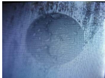
Dirty: Cleaning required
